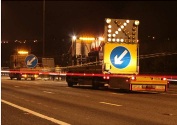
Installation of Temporary Traffic Management underway utilising two Impact Protection Vehicles (crash cushions) to protect the workforce during sign and cone deployment
